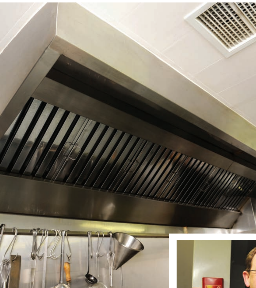
Extractor System installed by O'Leary Ventilation and Duct Cleaning Services in the kitchen of Lord Kenmare's Restaurant, College Street, Killarney. Photo by Michelle Cooper Galvin.
